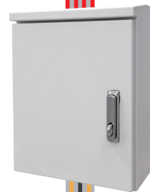
OS-210 Series Outdoor IP PoE Cabinet with Integrated Power and Battery Backup
